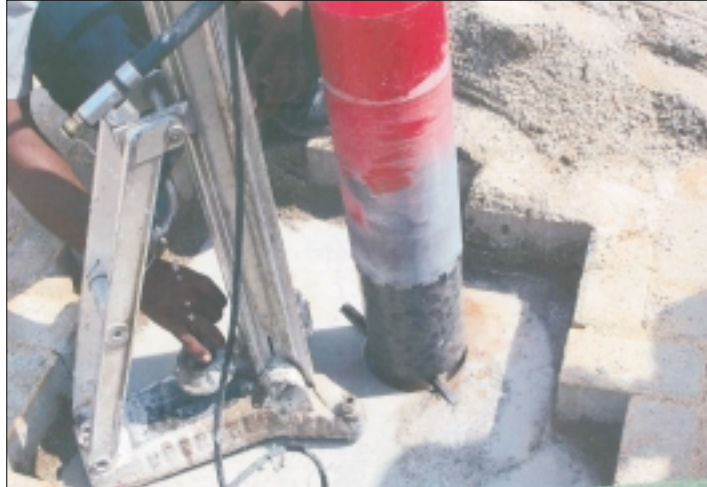
Core sample taken from Cement Concrete Pavement by Vigilance Team during Preventive Inspection in one of the projects.
